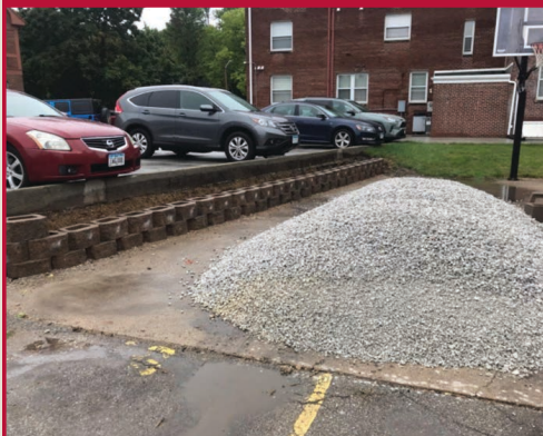
A significant effort was made to re-do the retaining wall by the basketball court.
